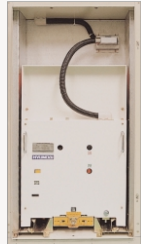
Circuit-breaker in the 'Service' Position
