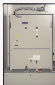
Circuit-breaker in the 'Service' Position
