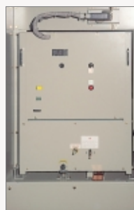
Circuit breaker in the 'Service' Position
