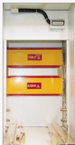
Circuit breaker Removed
