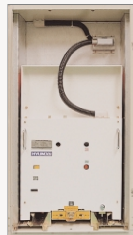
Circuit breaker in the 'Service' Position
