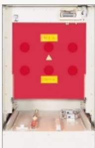
Circuit breaker Removed
